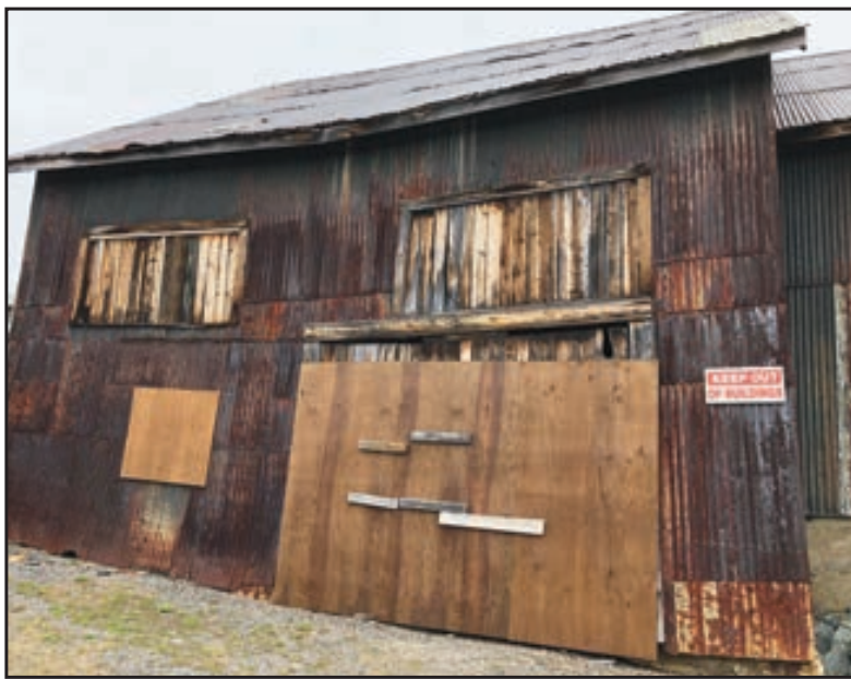
Forced entry into one of the buildings at the Right-of-Way mine site in Cobalt in late April received quick response by property owner Ontario Northland which has now boarded up access points to both buildings on the property. (Staff photo by Darlene Wroe)
