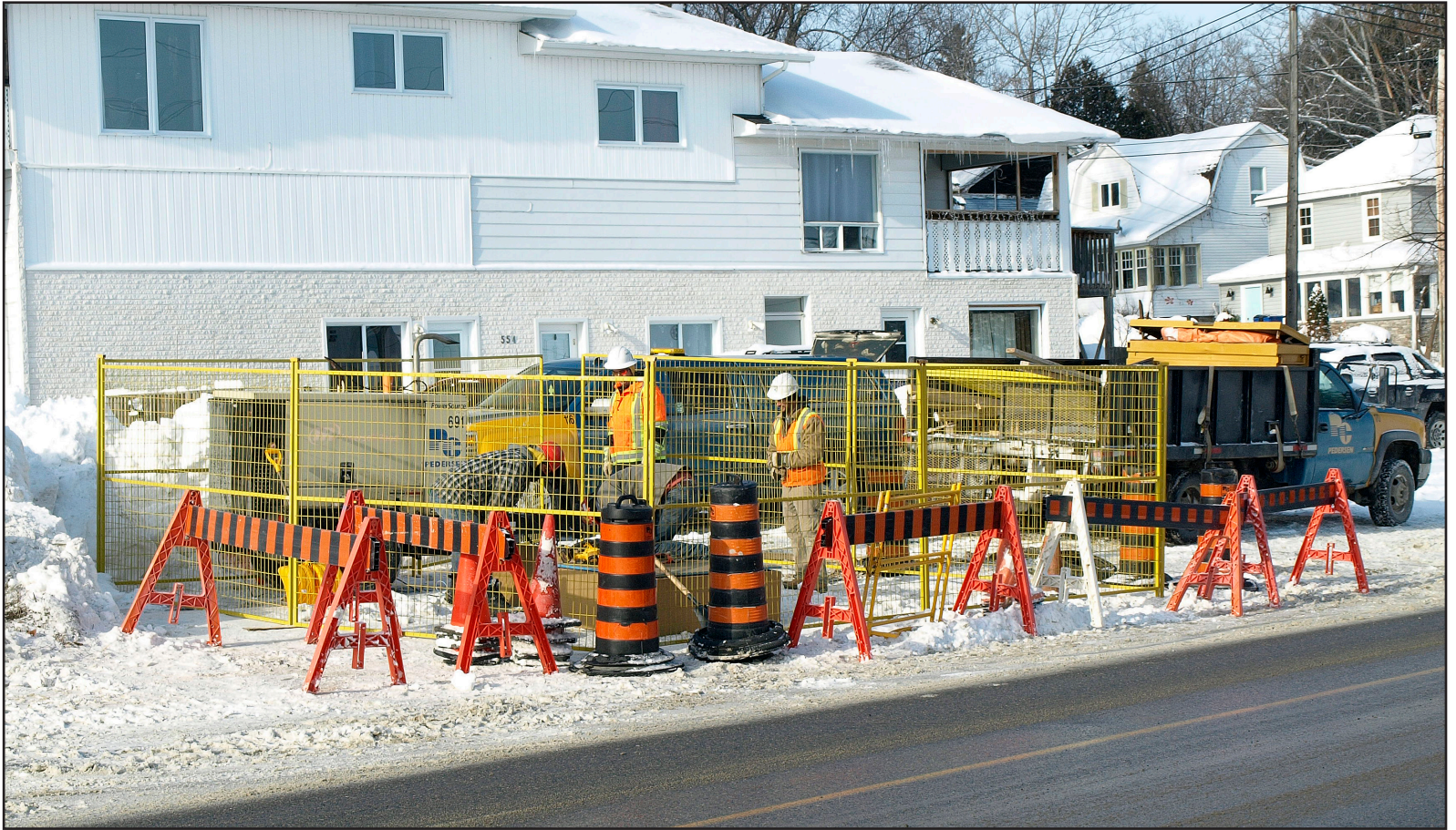
Workers were in downtown Haileybury late last week, where an underground utility vault was being vented after a hydrocarbon smell was reported in the area. The city has retained Story Environmental to assist with the investigation into the source of the odour. (Staff photo by Diane Johnston)
