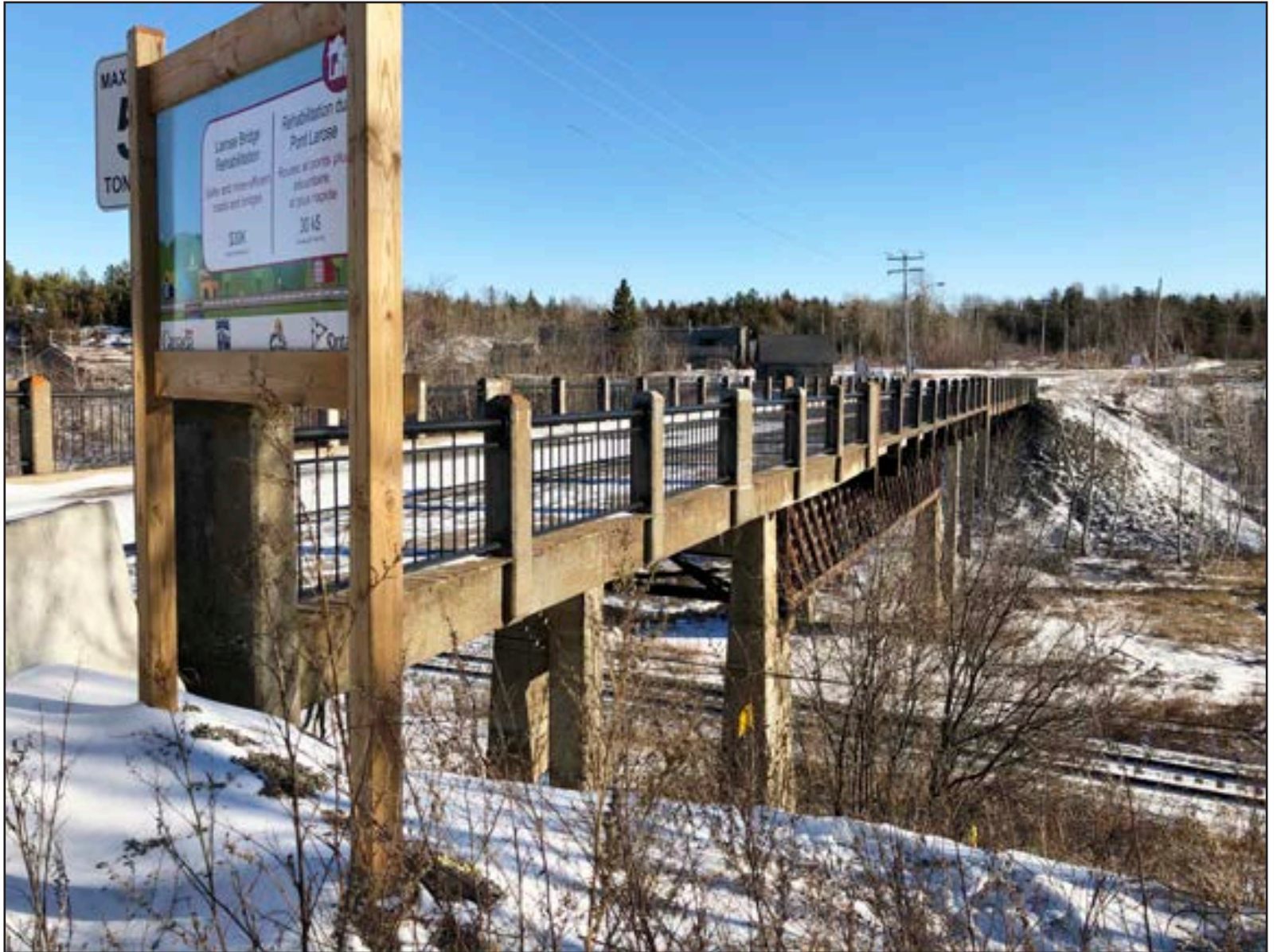
The Larose Bridge, which connects Cobalt and Coleman Township, will be torn down early this winter and a new replacement bridge will be constructed in its place over the course of 2021. (Staff photo by Darlene Wroe)
