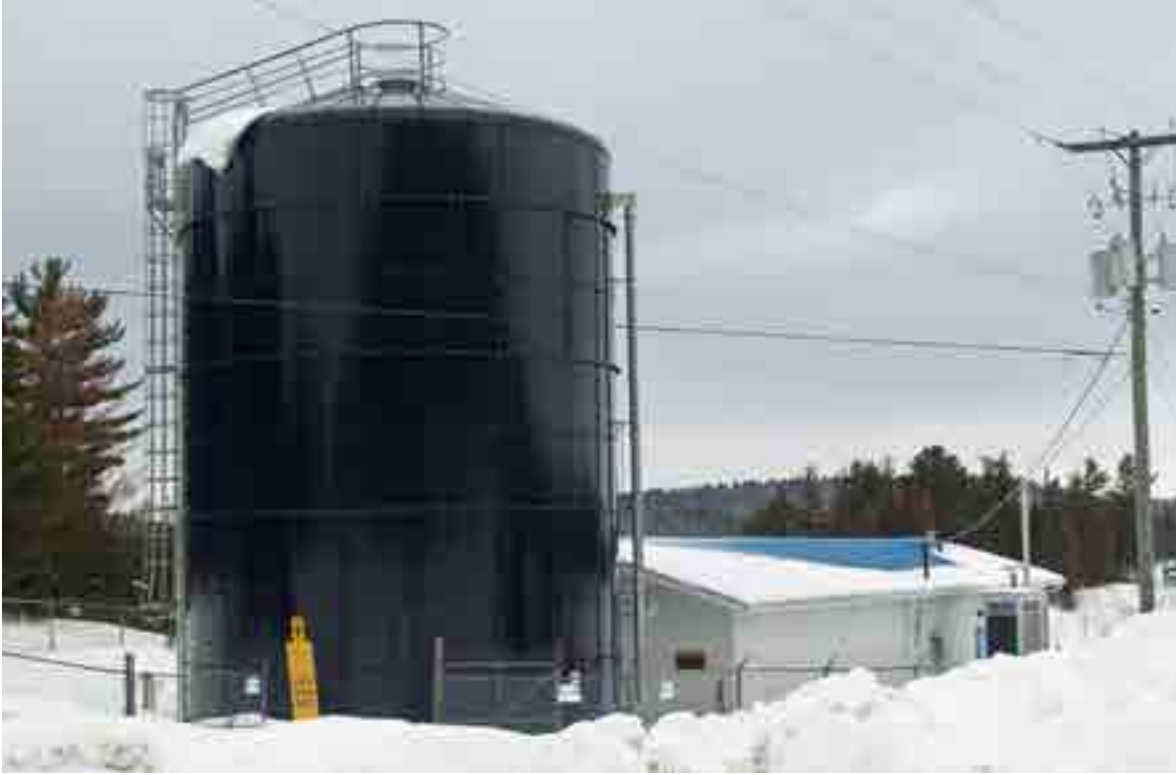
The water treatment plant and new holding tank addition in Coleman Township at Sasaginiga Lake. (Staff photo by Darlene Wroe)
