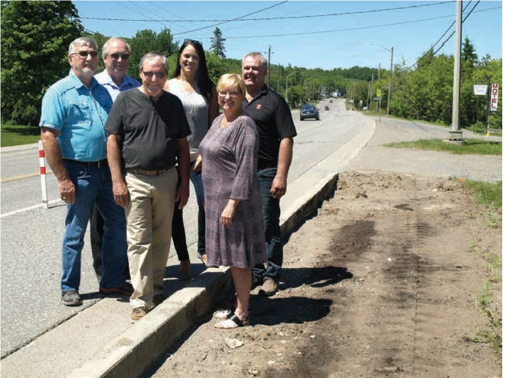
Representatives of Temiskaming Shores and STATO checked out the progress of construction that will relocate the trail off Lakeshore Road North, reopening a stretch of the roadway to year-round two-lane use. Seen at the site last week are, from left, Temiskaming Shores Councillor Doug Jelly, Mayor Carman Kidd, Councillor Danny Whalen, STATO's Linda St. Cyr, city recreation director Tammie Caldwell, and STATO's Tom Cambridge. (Staff photo by Diane Johnston)
